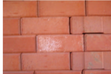
Plate 2: Solid interlocking blocks used in construction of analytical and materials laboratory, NBRRI, Ota, Ogun State Nigeria. Source: Field Survey (2007)
